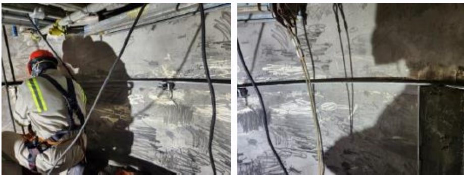
The supports for the new liquid and gas distributors are installed between beds #3 and #4
